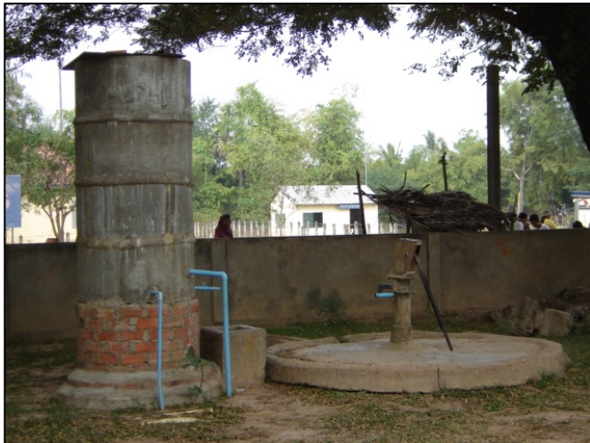
A locally constructed water system for providing clean water throughout the school
