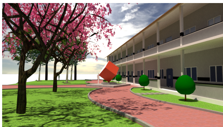
Renewed Modernization Efforts in Schools Get Under Way: Workers begin the emplacement of new ceilings at a dilapidated building at Akhea Mahsei PS in Kampong Speu (above); Idealized view of landscaping at Prek Leap HS in Phnom Penh
